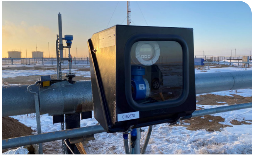
Flow meter into GRP ATEX enclosure (Kazakistan)
