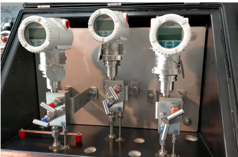
3 PT transmitters into GRP enclosures
