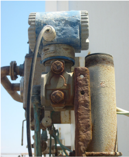
Transmitter not protected by GRP enclosures (Italy)
