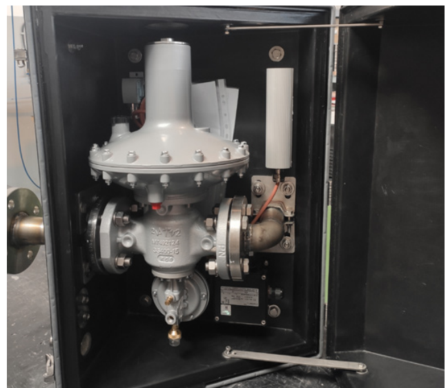
Valve installed into GRP ATEX enclosure
