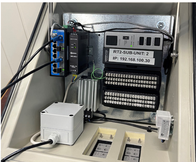
Data logger into GRP enclosures (Norway)
