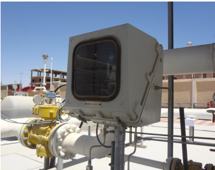
GRP enclosures installed at gas plant (Egypt)
